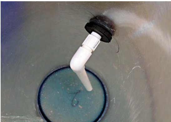
Figure 15. Since this piece is entirely internal and leakage is not a concern, you do not need to use Teflon tape or pipe dope
