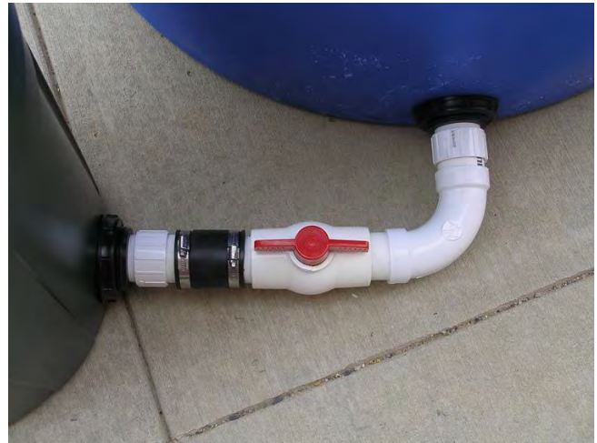
Figure 7. The completed plumbing assembly allows water to move from tank to pump
