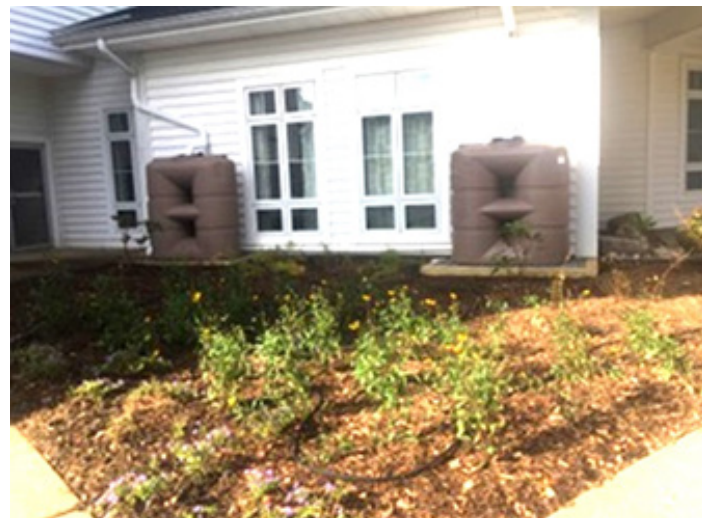
Gene McKenzie and crew of McKenzie Contracting, installed the Conservation Landscaping and Rainwater Harvesting project. Image source: Jackie Takacs.
