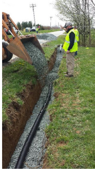
Marshall McSorley signals the backhoe operator on how much stone to place in the newly-excavated roadside bioswale. Photo Credit: Eric Buehl
